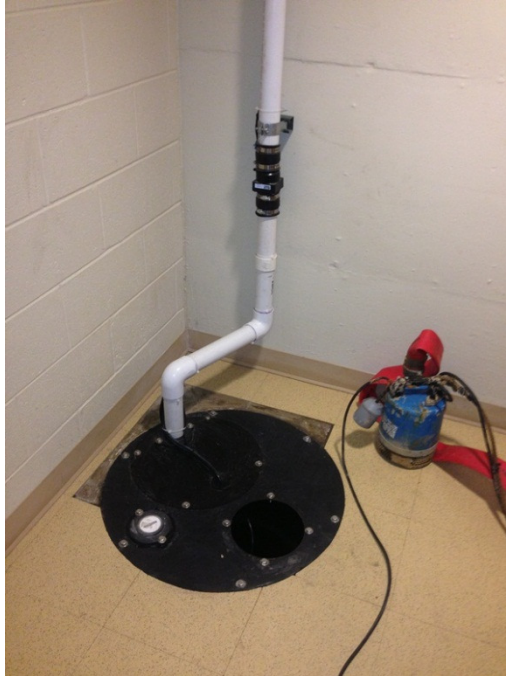
Photo 2.2-2 Westerly Sump Pump Structure with Secondary External Pump
