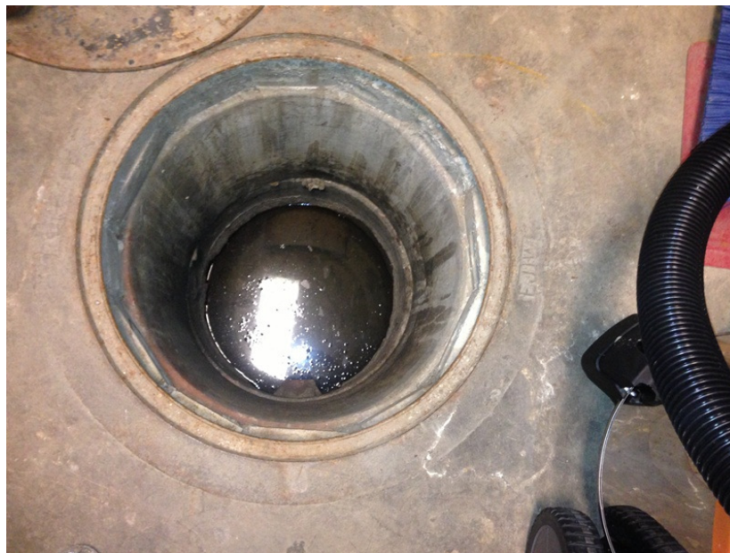
Photo 2.2-1 Central Sump (Wet System Operation)
